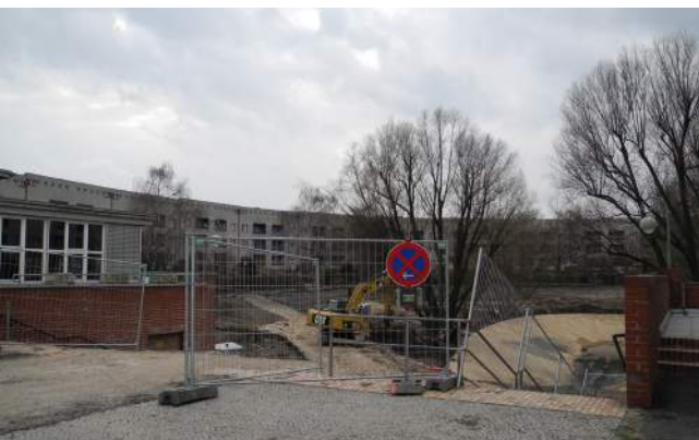
Figure 3: Work in progress on the restoration of the inner courtyard in Hufeisen (Photo: Iryna Shalaginova 2011).
